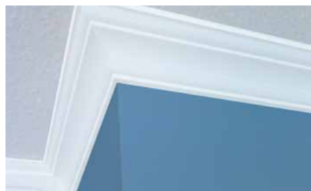
InvisiLight ILU Solution installed in a residence
